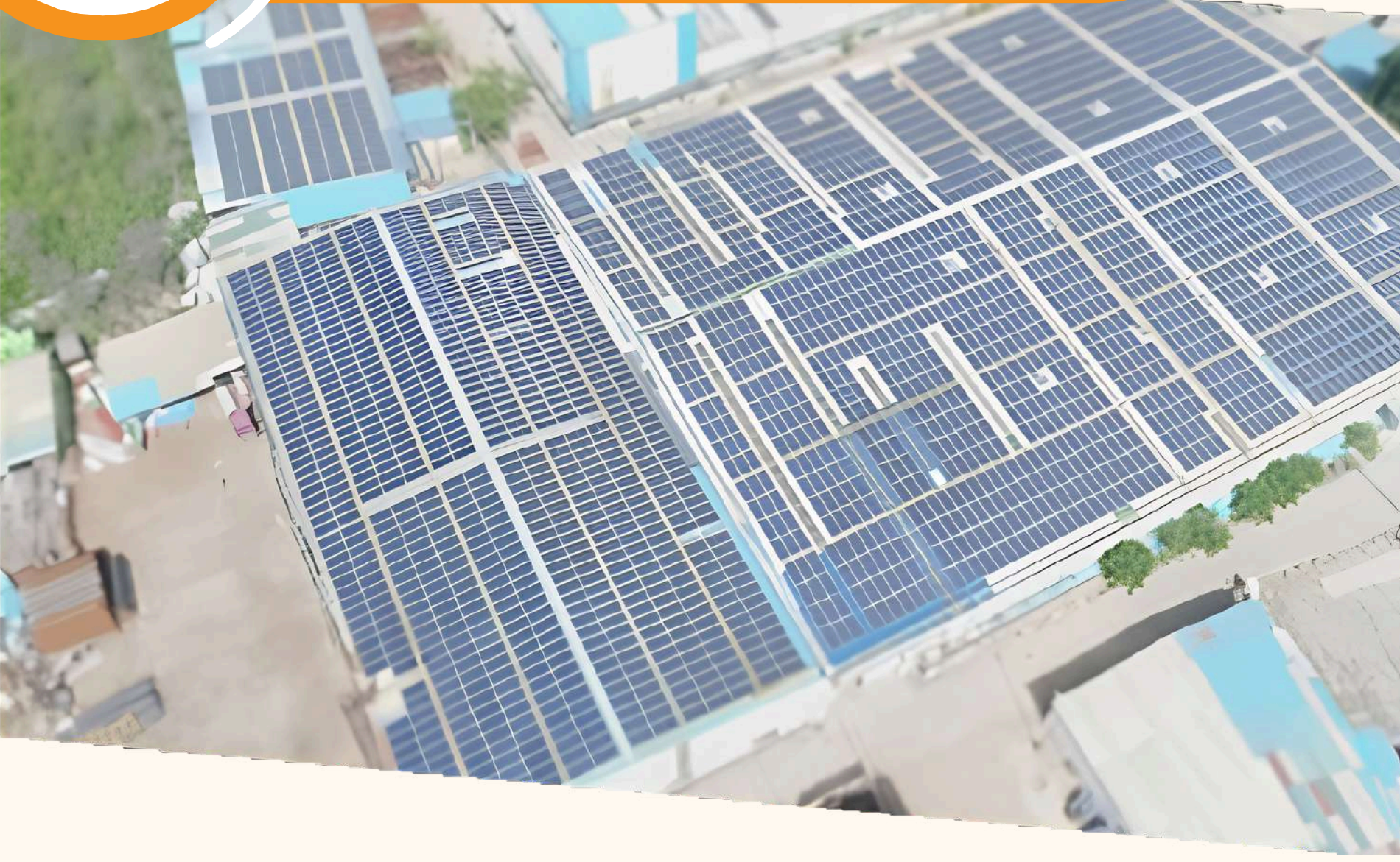
Himachal Pradesh 27MW
